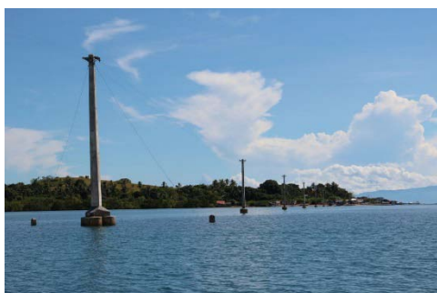
Electrification, Lapinig, Bohol
